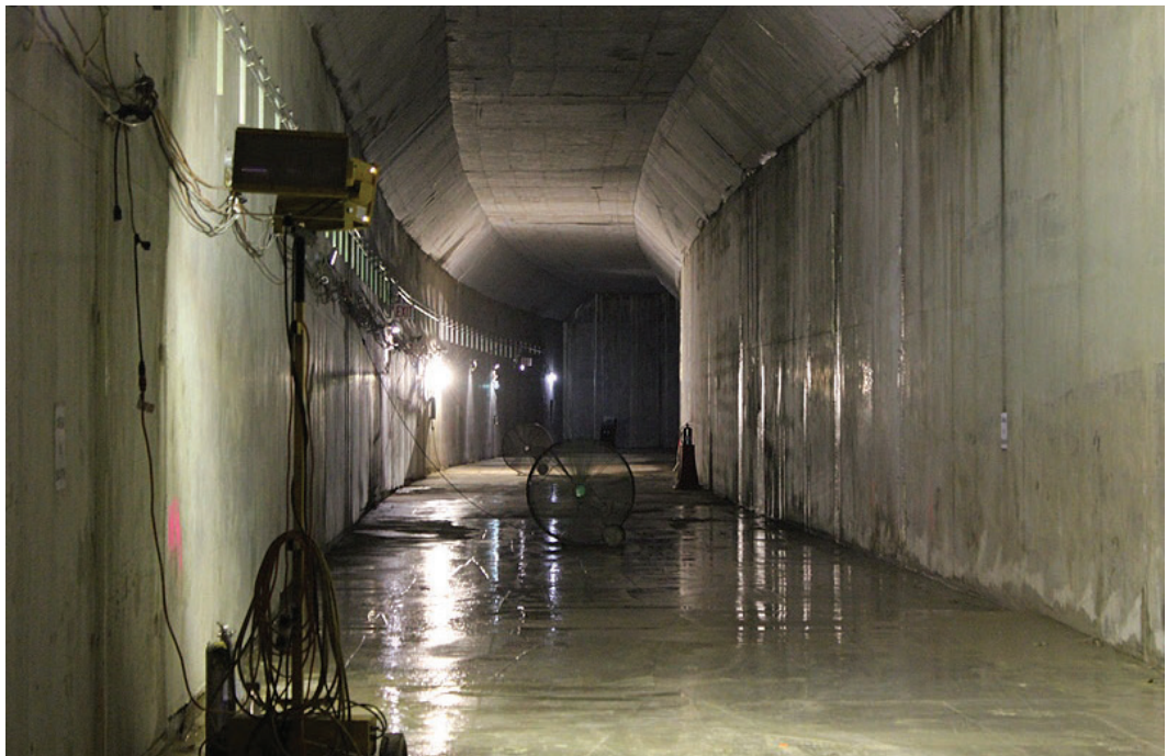
Sections 1 and 2 of the Hudson Yards Concrete Casing have been completed to preserve a right-of-way under Hudson Yards.
