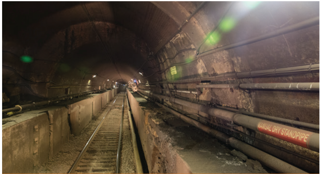
Damage in the North River Tunnel
