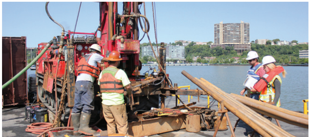
Rock and soil samples are being taken to better understand the underground conditions prior to tunnel construction.
