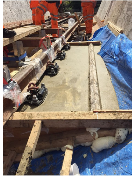
Figure A10.1 –Surface mock-up of the planned rail replacement for Baker Street to Finchley Road underground stations.
