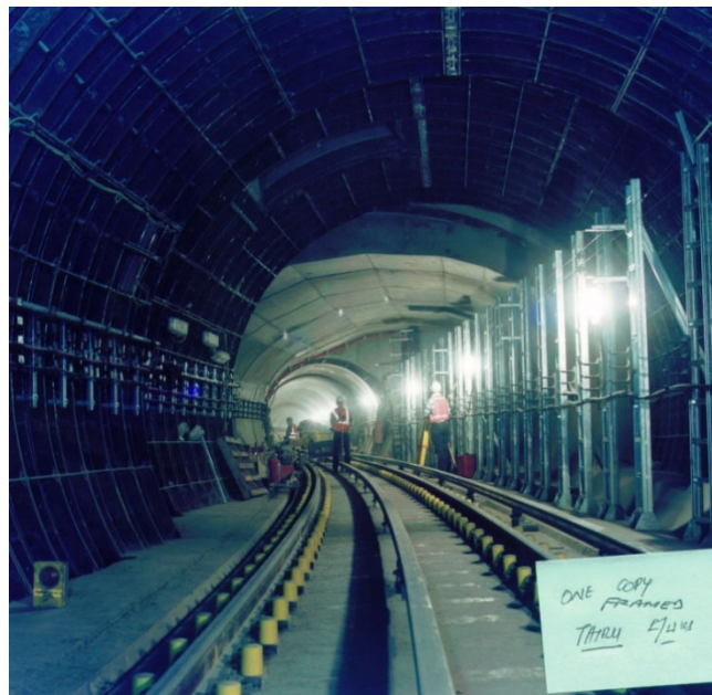
Figure A10.5: London Bridge Station Northern Line Link under the river Thames
