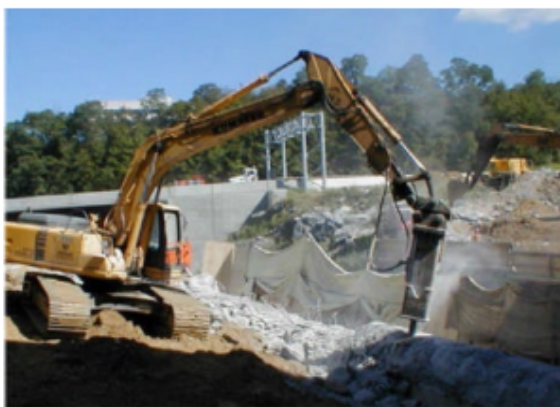
Excavator equipped with an enclosed cab and hoe-ram demolishing a concrete wall.
